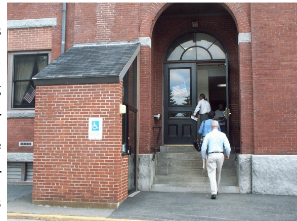
Figure 4: Abandoned wheelchair lift enclosure.
