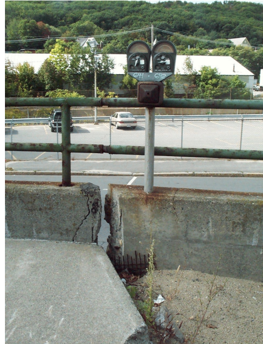
Figure 7: Crack between garage and on-grade parking lot.
