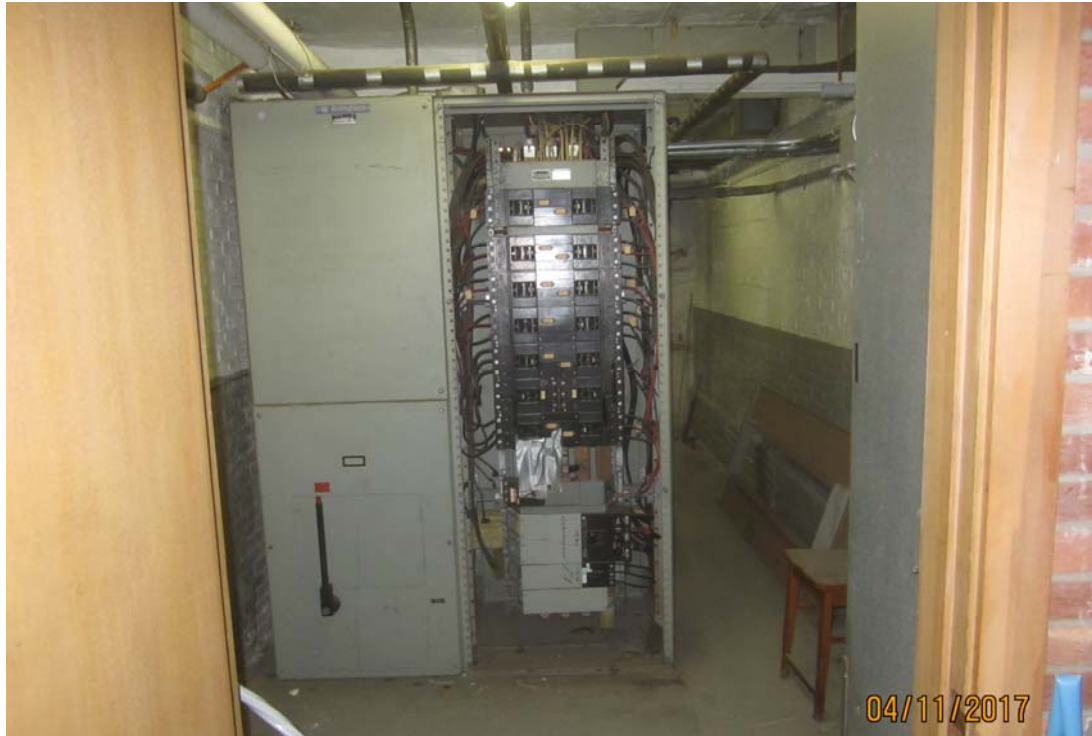
View of existing electrical room
