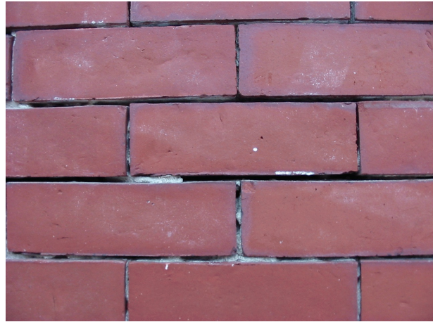
Figure 8: Open mortar joints.
