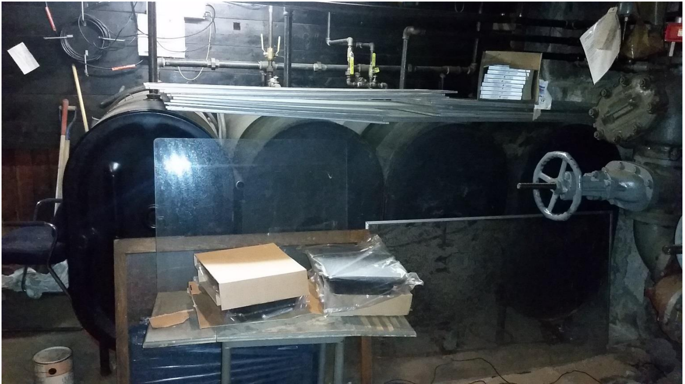
Photo 47 Basement – heating oil storage tanks
