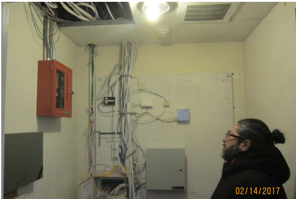
View of bank building existing electrical closet
