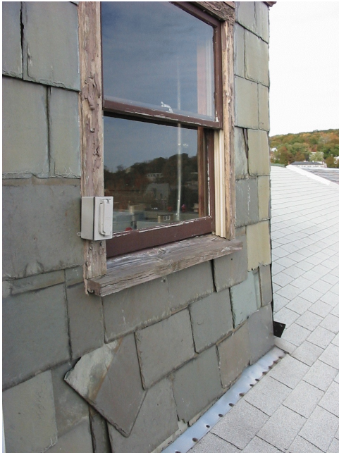
Figure 12: Falling slate tiles on dormer.
