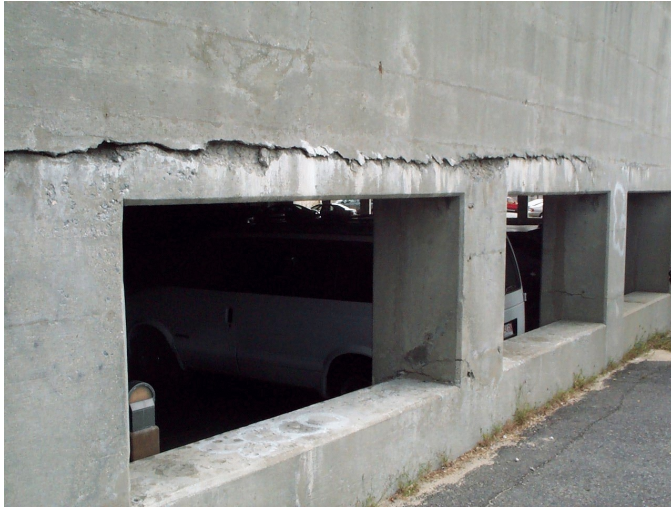
Figure 6: Cracks in spandrel beam of garage.
